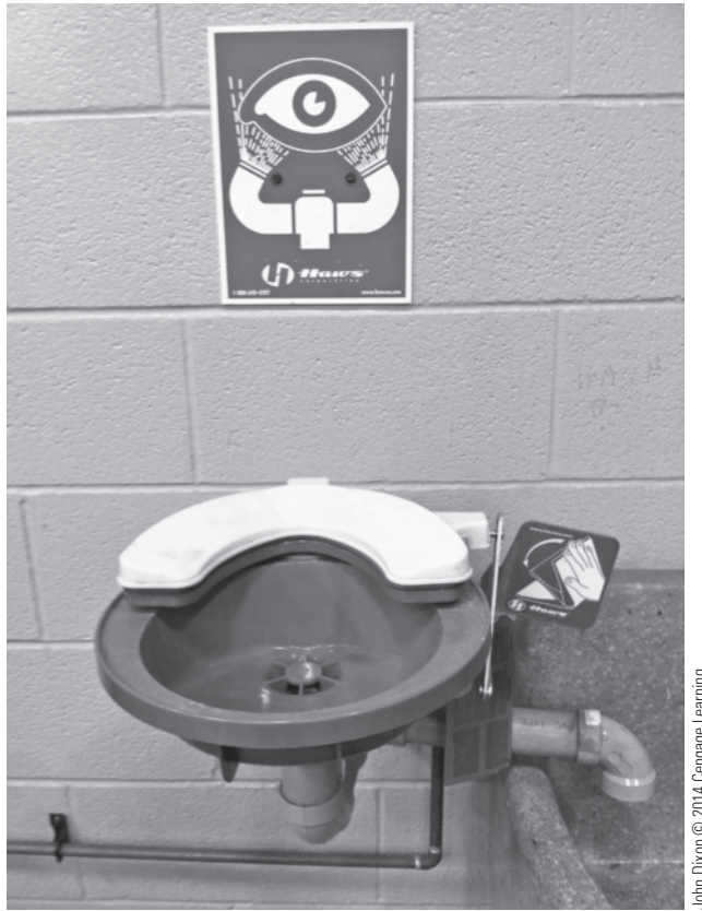
Figure 2-9 Eye wash station.
