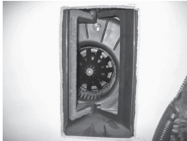
Figure 9-11 The recirculation door is open, allowing fresh air to be introduced into the HVAC.
