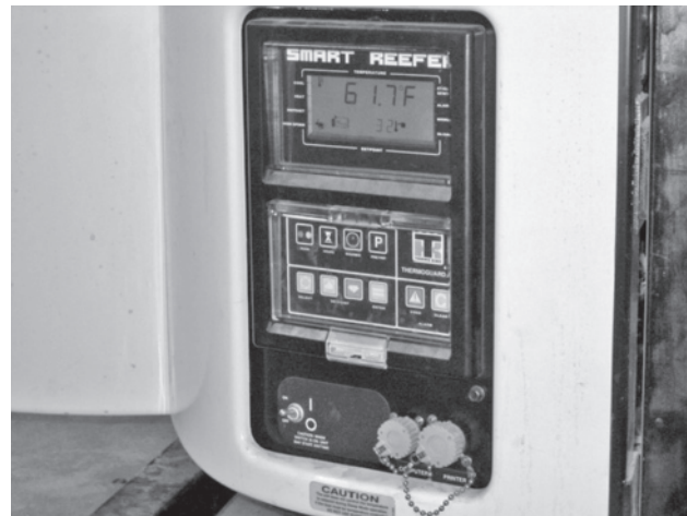
Figure 13-5 A microprocessor-controlled thermostat.
